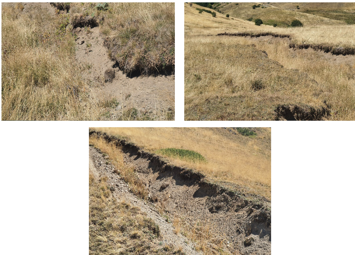
Figure 32. Erosion signs noted within Korabi nature park
